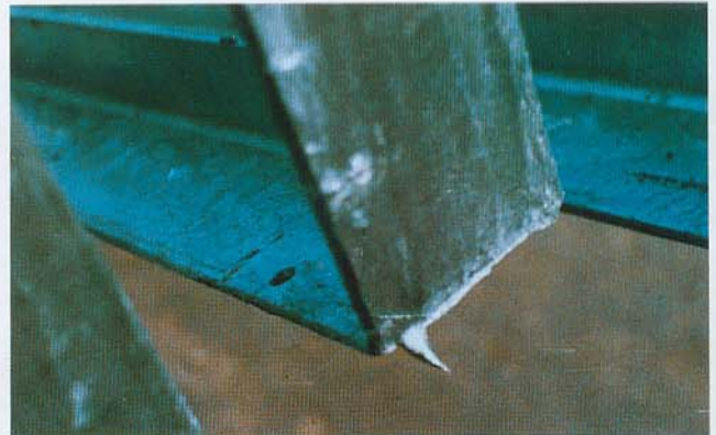
Fig. 2: Sharp zinc spikes which could cause injury must be removed
