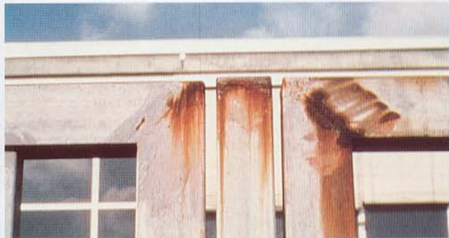
Fig. 4: Corrosion resulting from an incorrectly repaired weld
